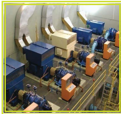
Misverstand pump station
